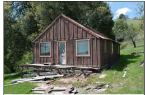
Wilson Ranch, 2010 Front Porch Missing
